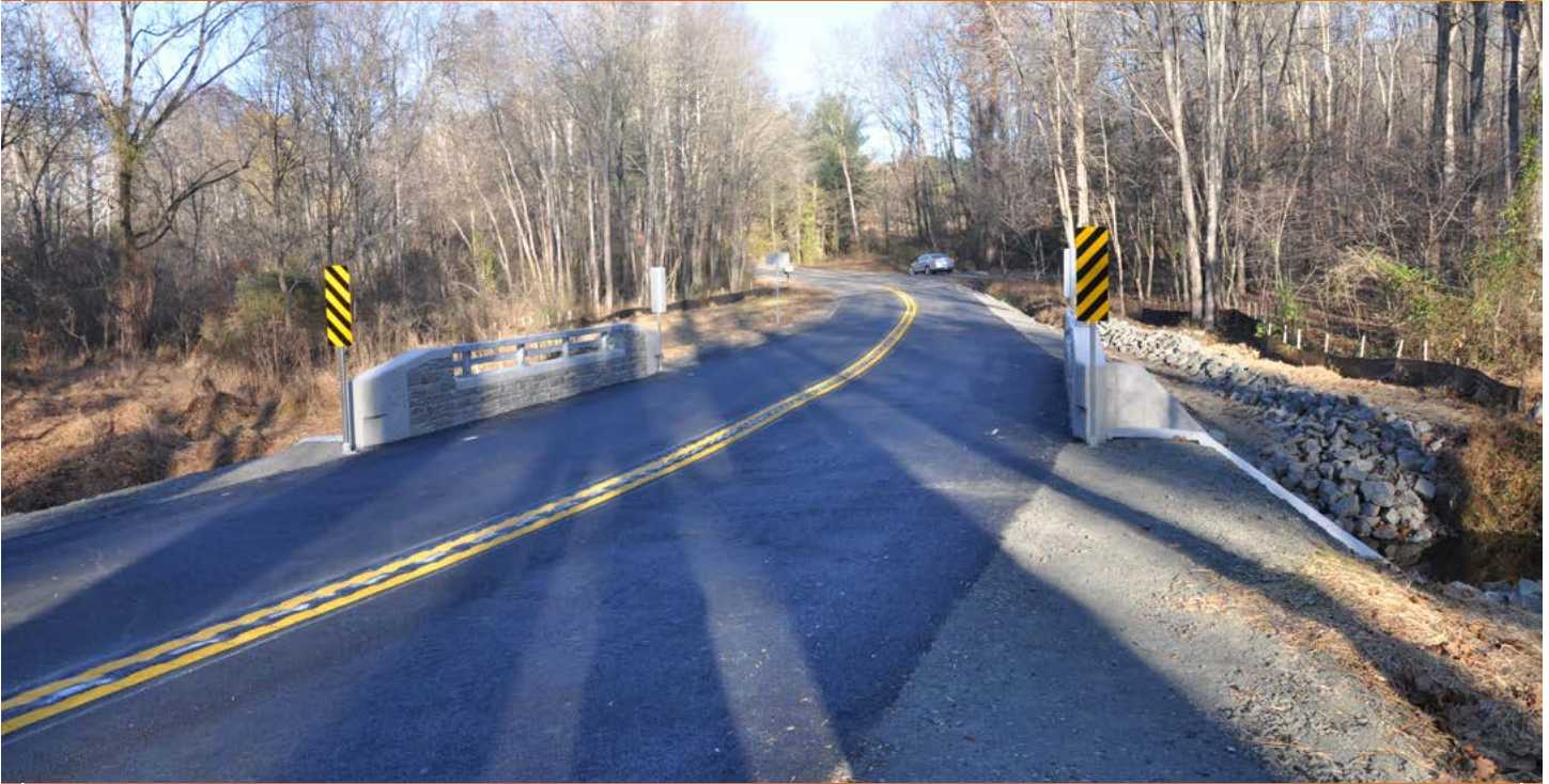
Replacement of the Route 647 bridge over the East Branch Thumb Run was completed Nov. 9.
