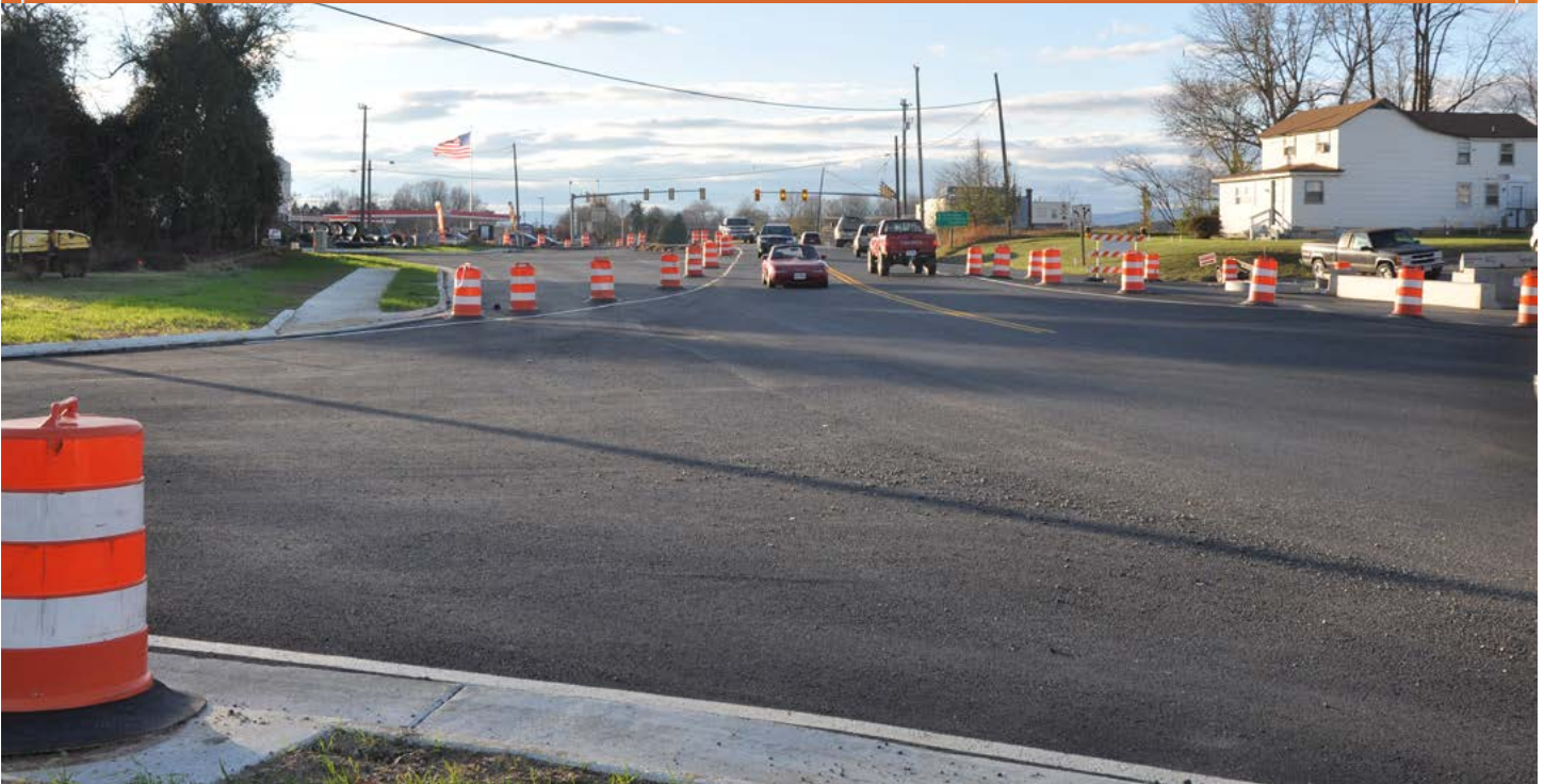
Construction for the road improvements at U.S. 33 and U.S. 29 in Ruckersville is under way, with anticipated project completion in July 2023.
