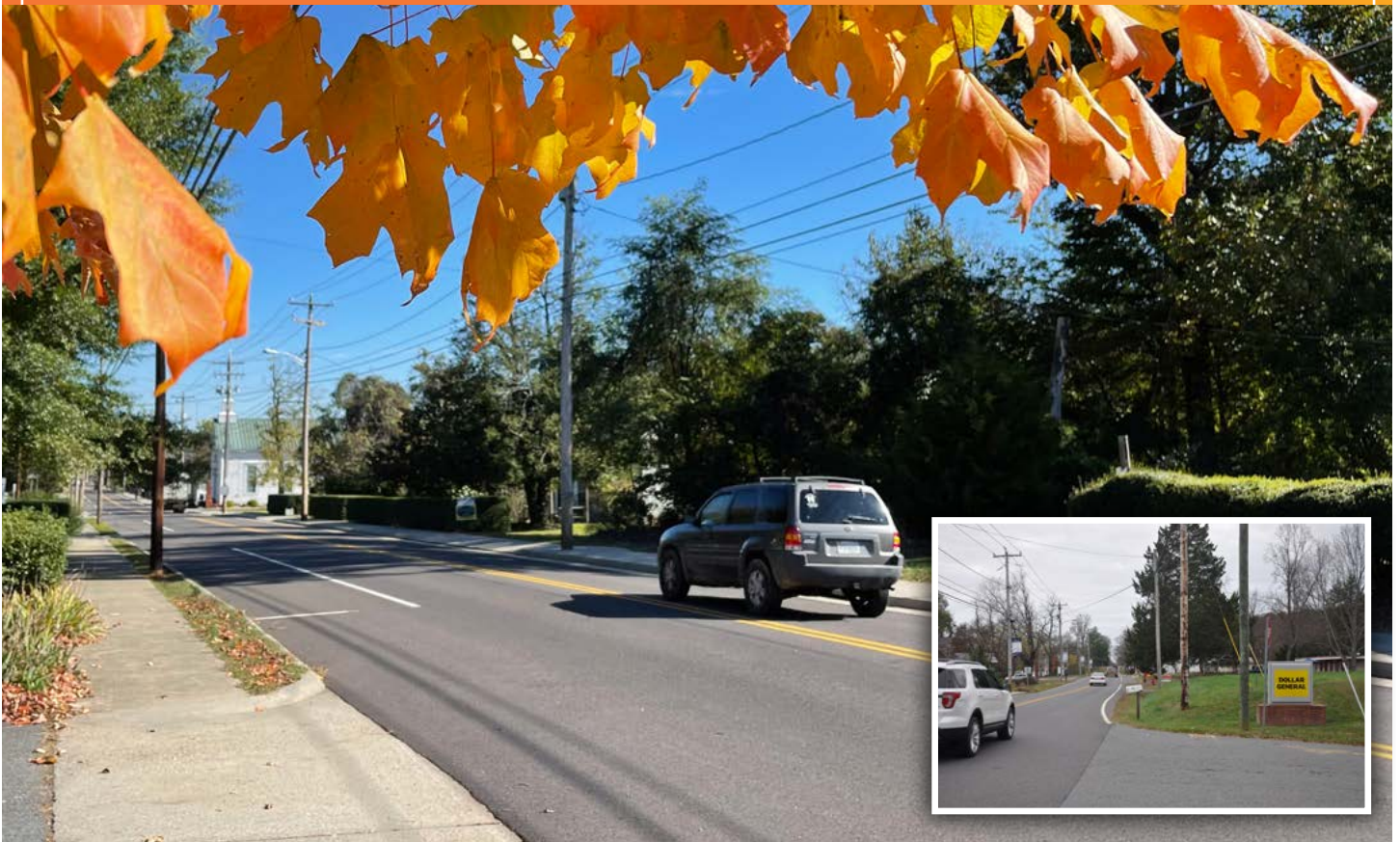
A sidewalk extension project on South Main Street in the town of Madison will enhance pedestrian access just as the color-changing leaves enhance the street's beauty each fall.
